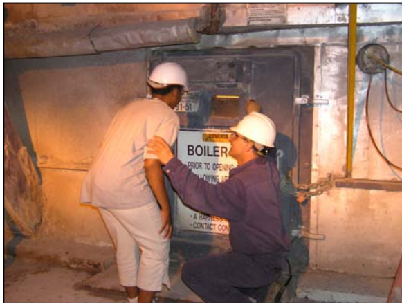
Peering inside the furnace at the Incinerator
