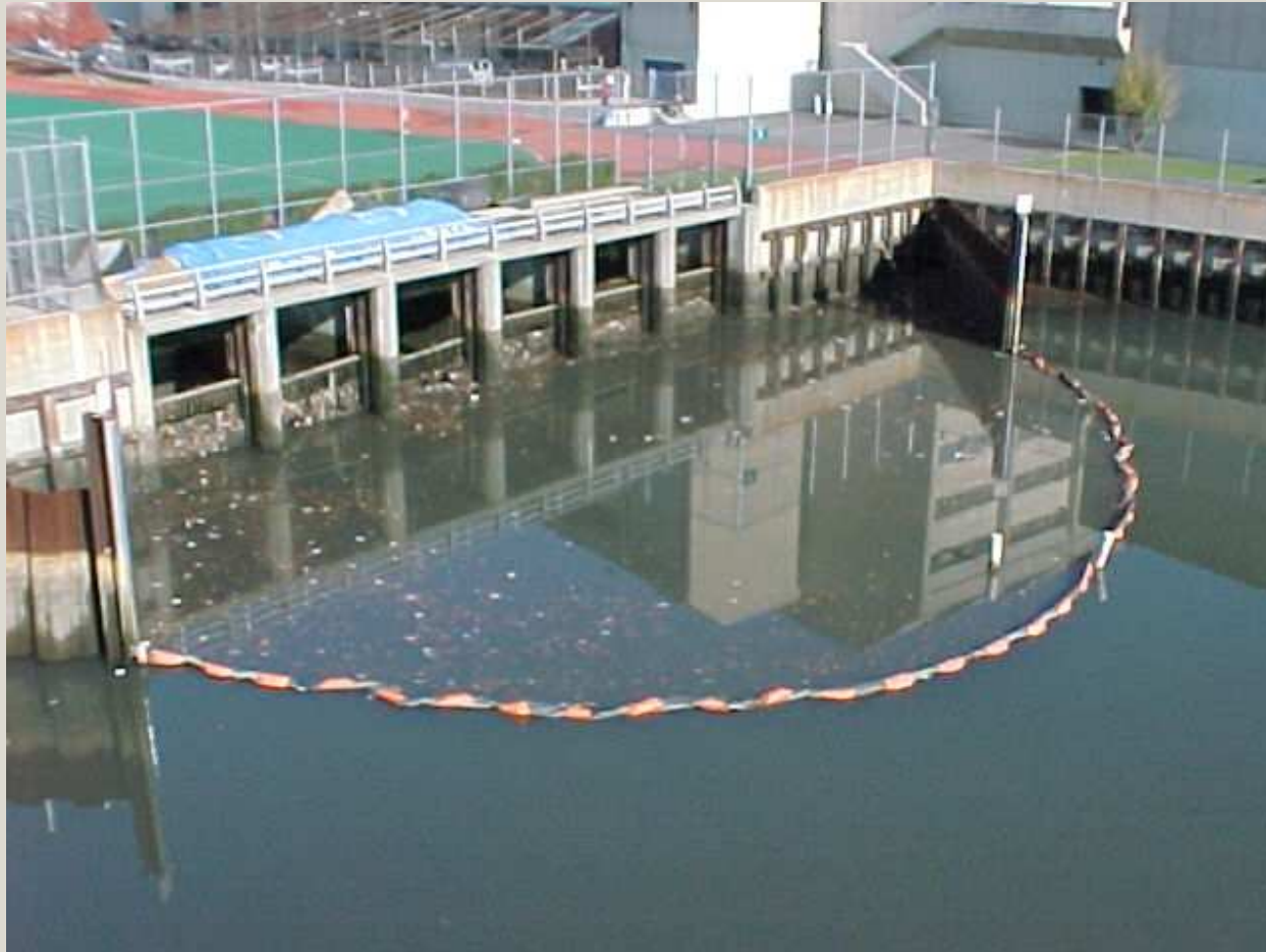
Simple Containment Boom at the headwall of a CSO outfall in Westchester Creek
